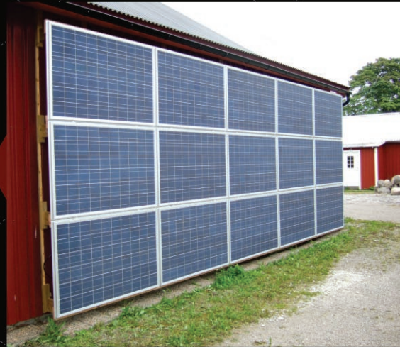
Involar Instalation - Sweden
