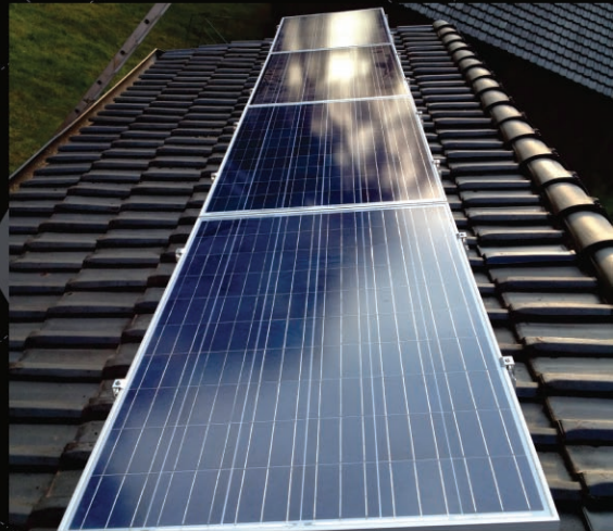
Involar Instalation - Germany
